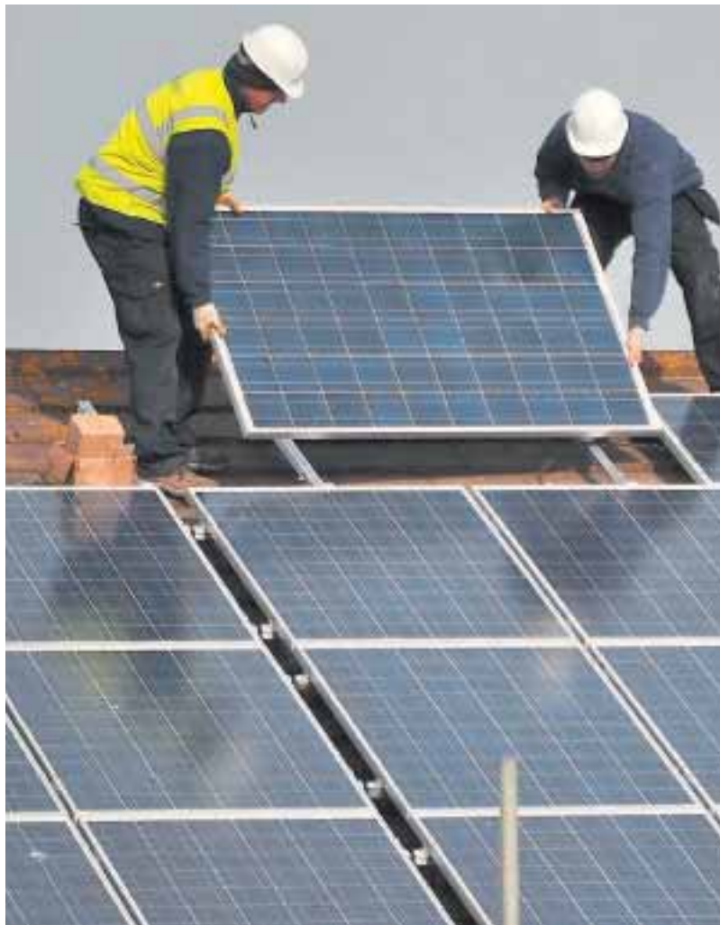
Work on covering the roof of Ashford's Civic Centre with 180 solar panels has nearly been completed, for the full story see below.
